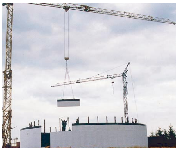
An element lined with Formtex ® is hoist into place by a tower crane.
