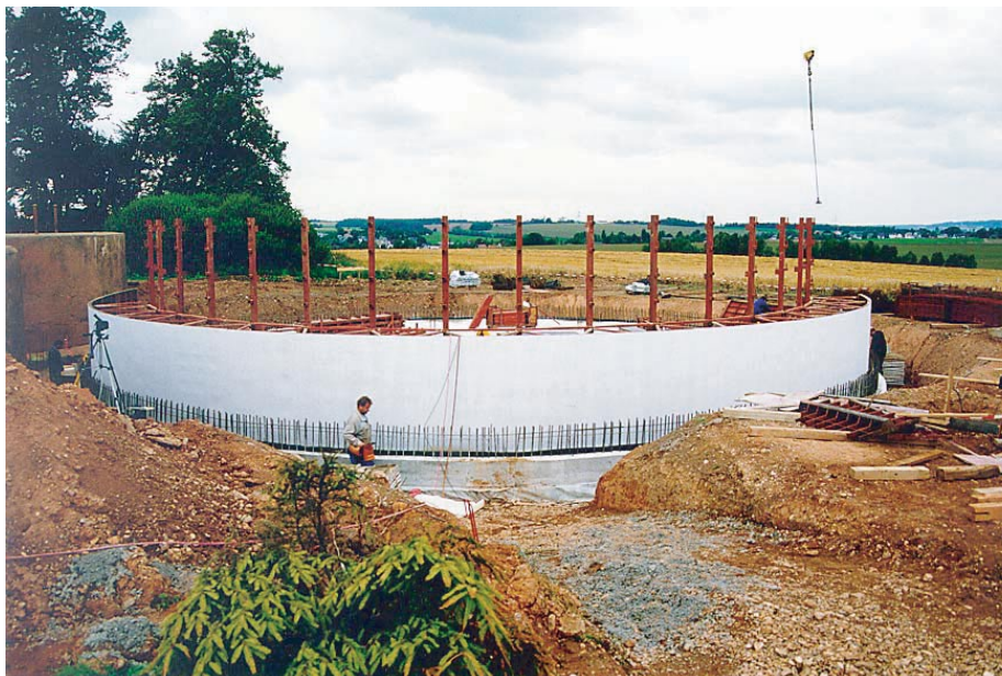
Drinking water tank before casting. The formwork elements have been lined with Formtex ® .
