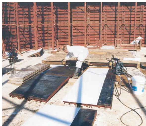
Glue is sprayed onto a formwork element and a length of Formtex ® is unrolled.
