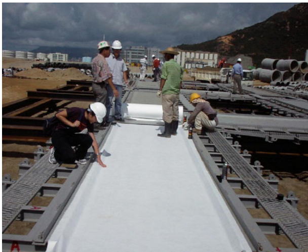
Figure 4. Formtex is installed on the base of the formwork for the beam.
