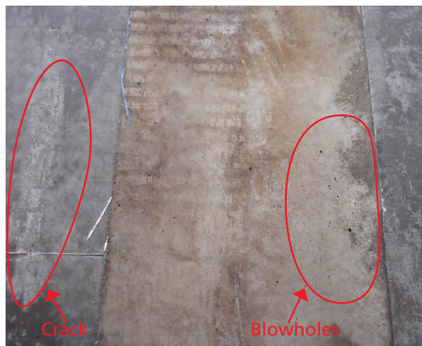
Figure 3. Achieved concrete for competing product (Left), without formliner (middle) and Formtex ® (right)
