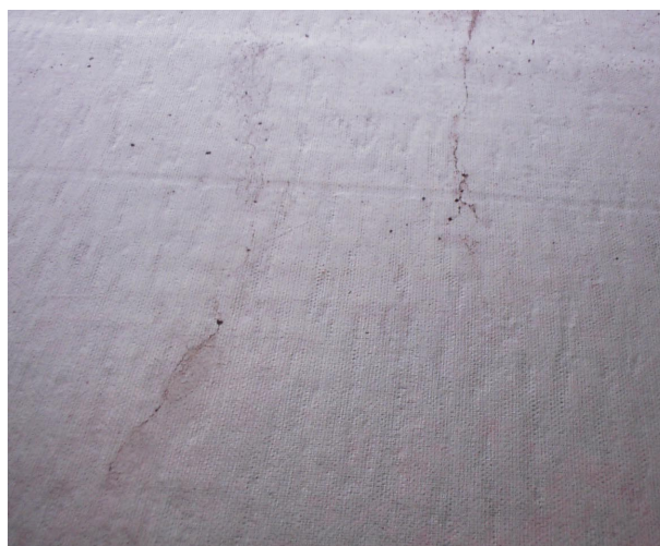
Figure 7. Several cracks in the surface of the test of the competing product.
