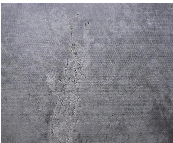
Figure 6. A large crack in the surface of the test of the competing product.
