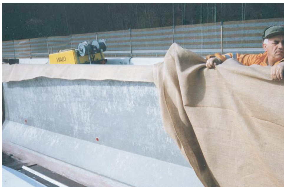
The finished parapet - Ready to use without any kind of after treatment.
